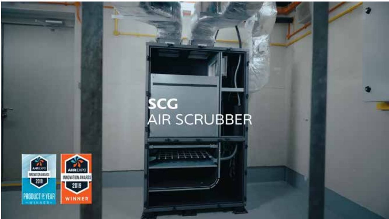
➤ SCG air scrubber, an innovative energy-efficient waste air treatment system
